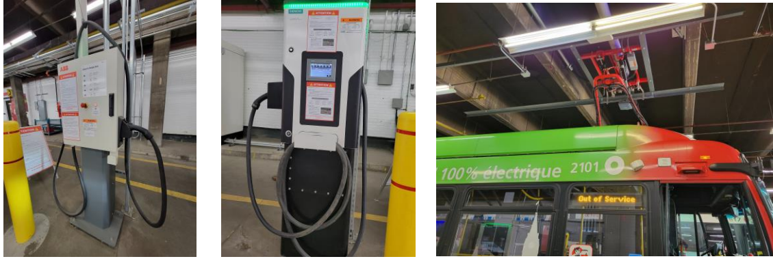
Figure 23: OC Transpo's electric bus Charging Systems
