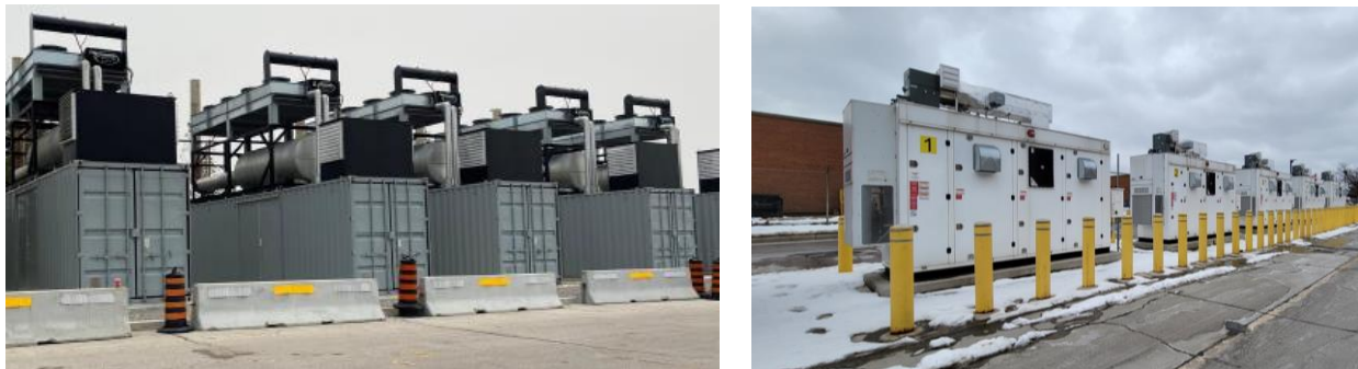
Figure 5: Arrow Road garage backup system (left: natural gas generators, right: batter energy storage system)
