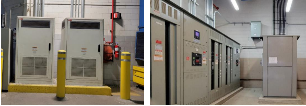
Figure 4: Example rectifiers 10 (left) and charging equipment panel (right)
